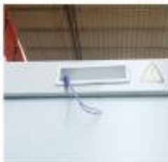
External main power supply
